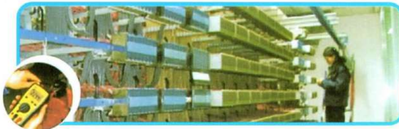
How to find the wire from among so many wires? It is so slow by using a multimeter.
